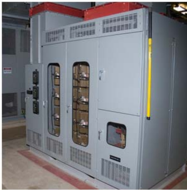
Power equipment at Metro's White Flint station
